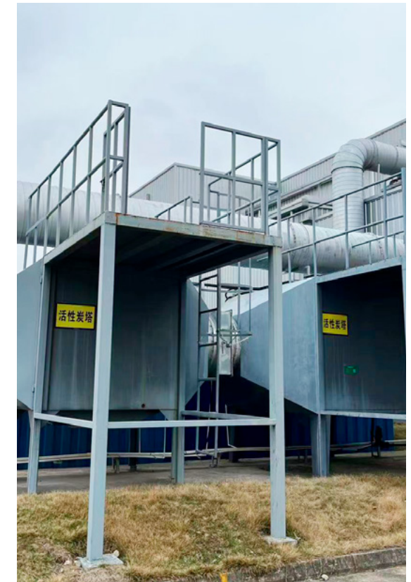
Double activated carbon facility at GC Suzhou
