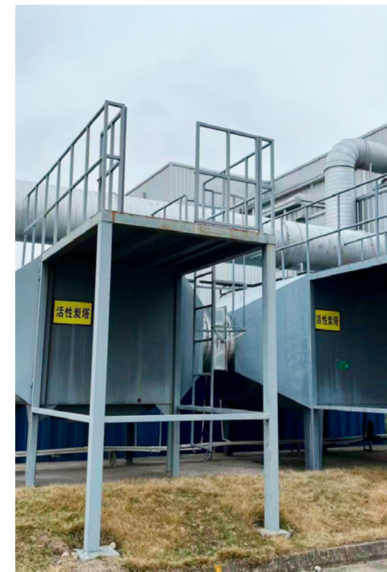
Double activated carbon facility at GC Suzhou
